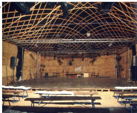
Gridshell roof over the Menteatrál theatre in Neratov, interior view POLÁČEK V., POKORNÝ V., Recycled Theatre, Praha: Grada Publishing a.s., 2015, page 309-310, ISBN: 978-80-247-5751-3
